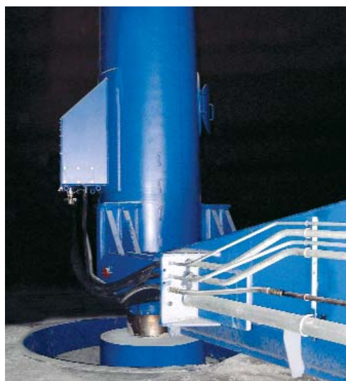
Bridge hinge and electrical transfer
