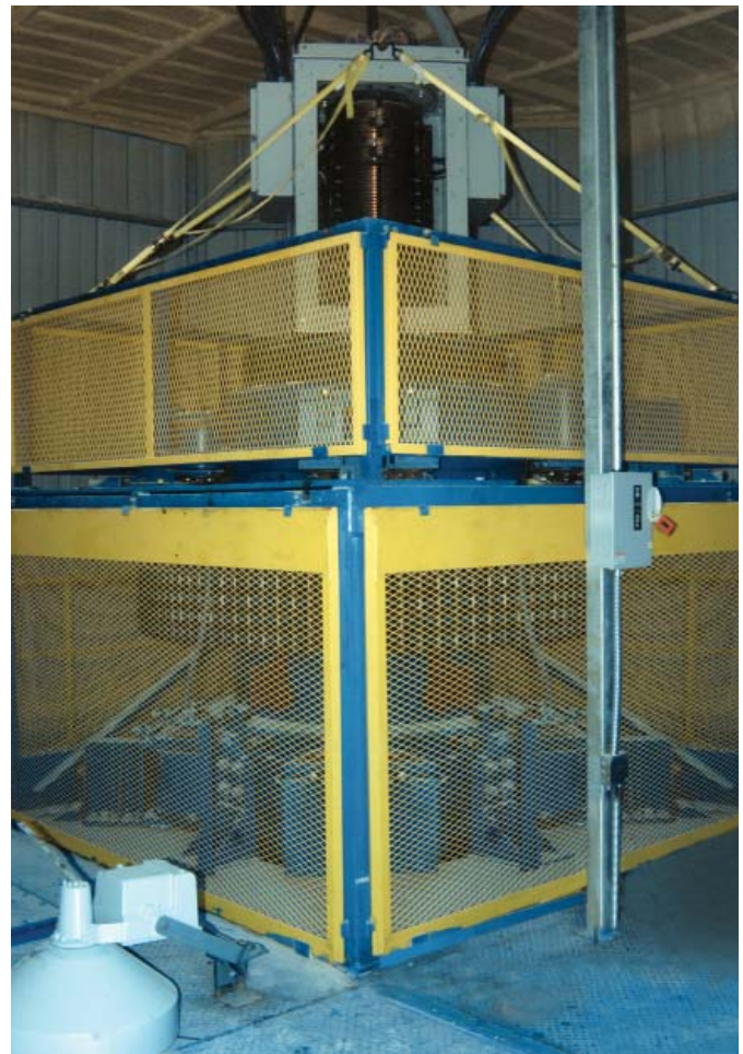
Column drive equipment and enclosed electrical slip ring assembly.
